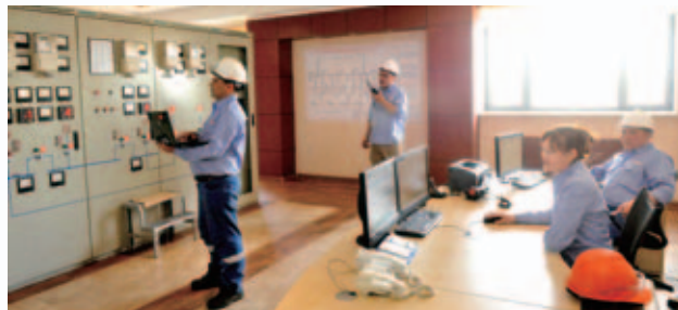
Dispatch center of the UHG Power Plant
